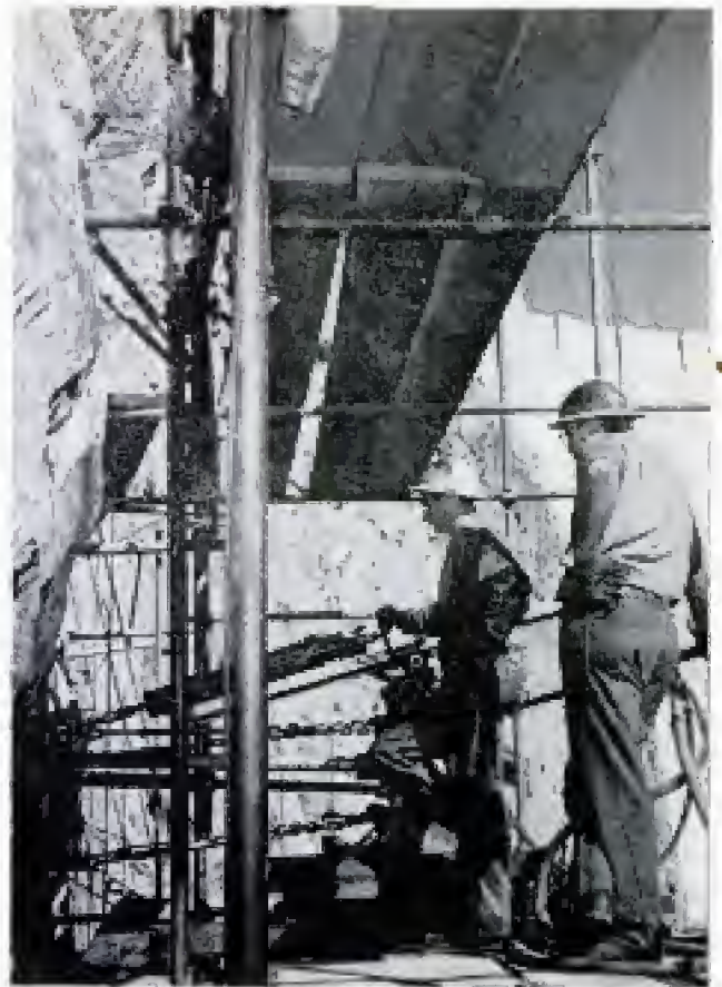
Drill grinds away to cut a hole in the slab. Holes were drilled 13 feet into solid abutment behind slab
